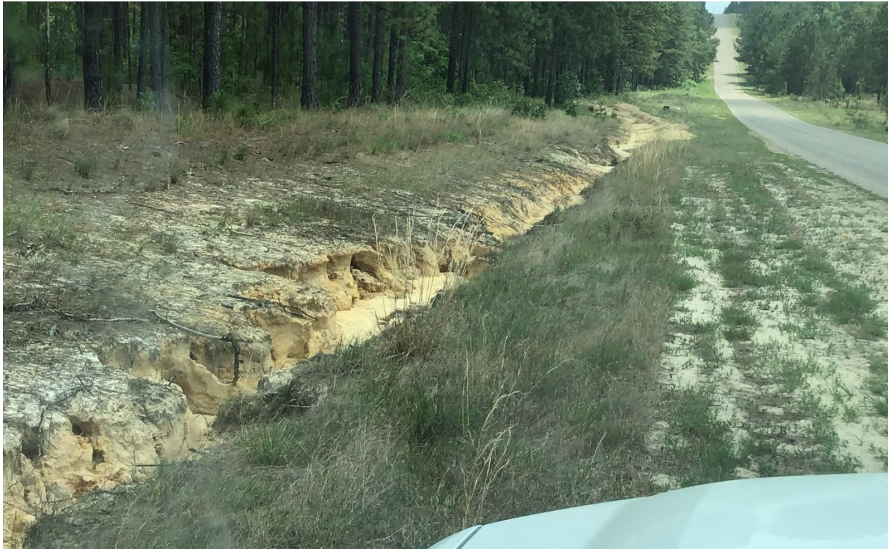
Ditch Erosion on King Road
